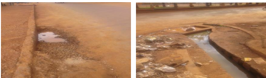
Figure 5: Poor Maintenance: resulted in eroded pavement & blockage
