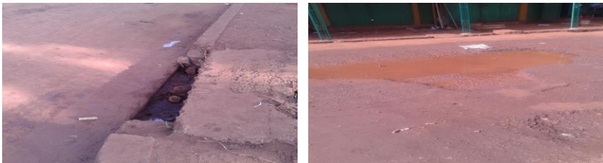
Figure 3: Poor maintenance: - resulted in Potholes & Failed Manhole
