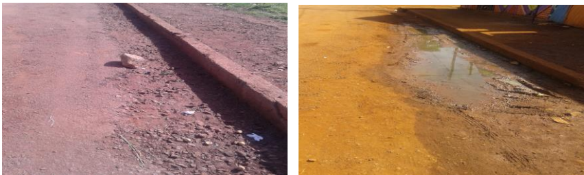
Figure 4: Poor Maintenance: - resulted in Edge Failure & Sediment Accumulation
