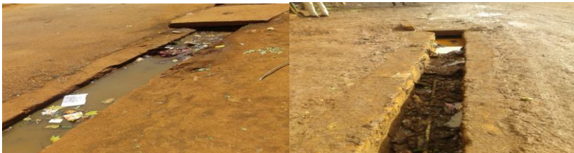
Figure 2: inadequate drain size accompanied by water logging
