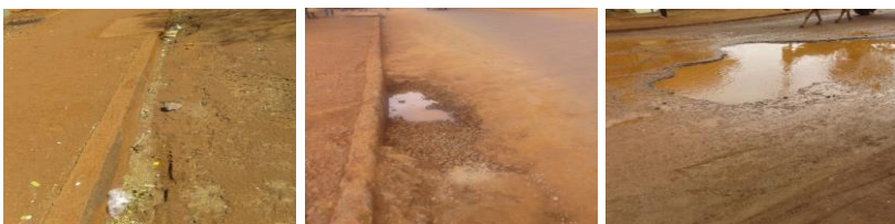
Figure 6: Severely failed edges and formation of potholes
