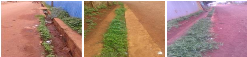
Figure 3: Collapsed & vegetated concrete drains
