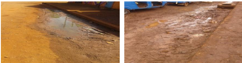
Figure 7: Silt & mud pumping on road pavements
