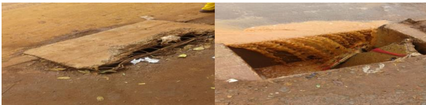
Figure 4: Failed manholes of side drain due to poor maintenance
