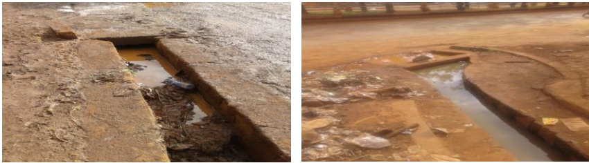
Figure 5: Blocked drains at Dead Ends
