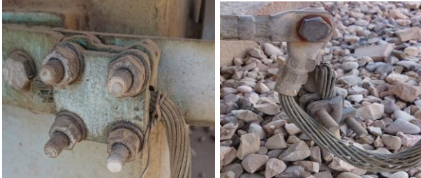
Figure. 8. The oxidation and reduced quality of Havanirooz Power Station earthing system
