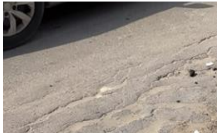
Image 04 – Isolated cracks in loco
