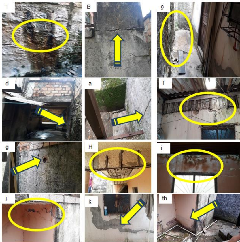
Figure 5 - Identification of pathologies in the structure of the residence
